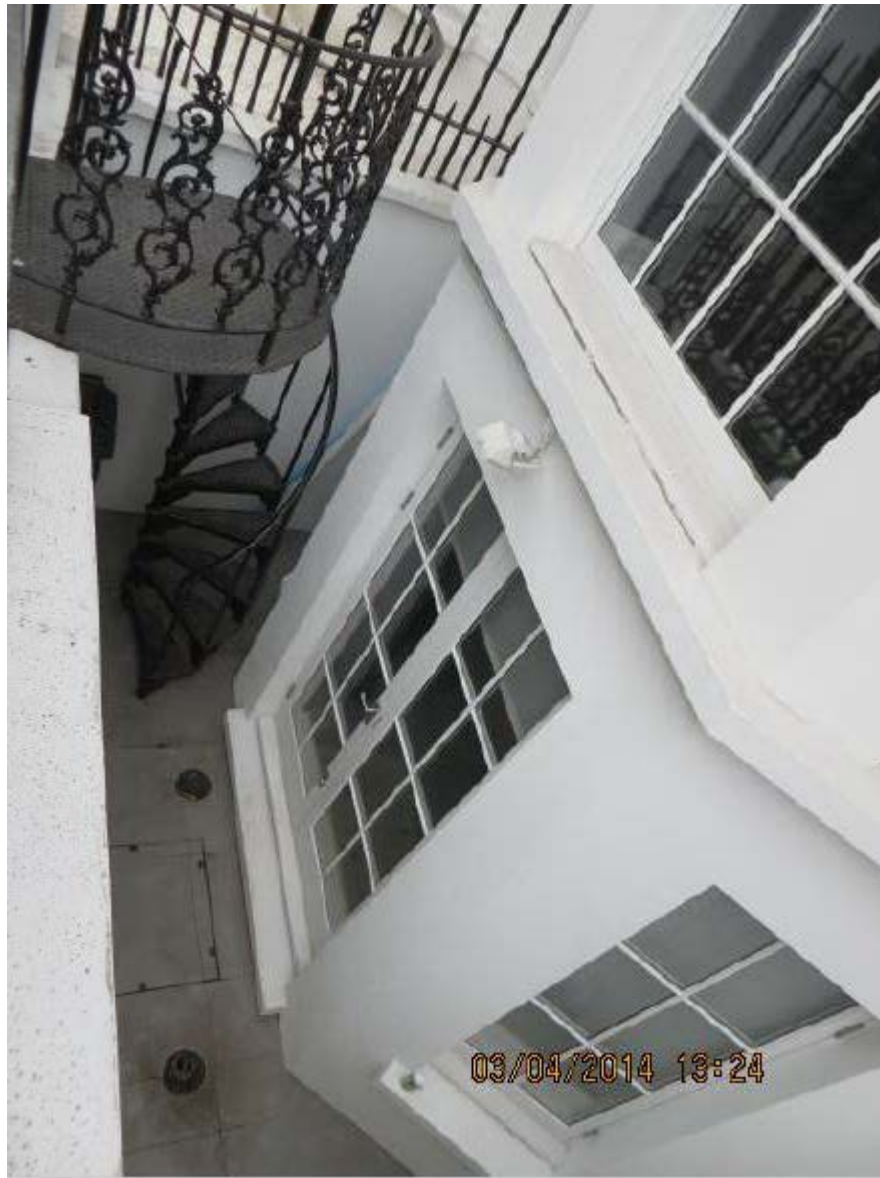
Existing unauthorised front lightwell to be covered over in Application 2.
